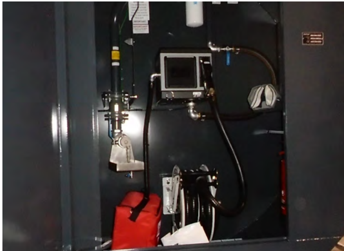
PIUSI FUEL MANAGEMENT SYSTEM INSTALLED IN BULK DIESEL TANK
