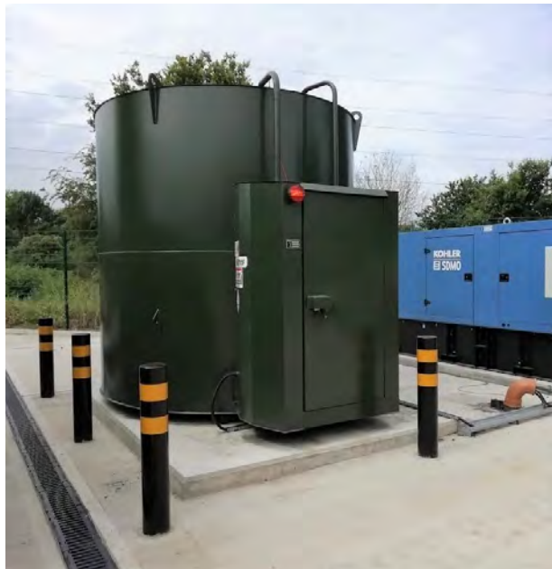
12,500 LITRE VERTICAL BULK DIESEL TANK
