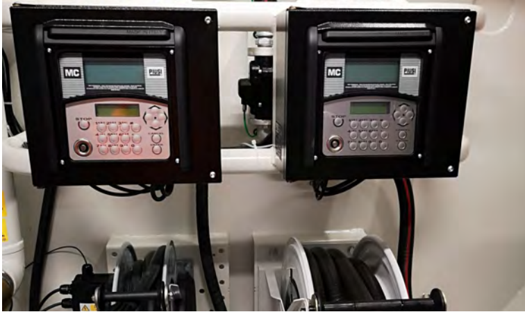
TWIN PIUSI FUEL MANAGEMENT SYSTEM INSTALLED IN BULK DIESEL TANK
