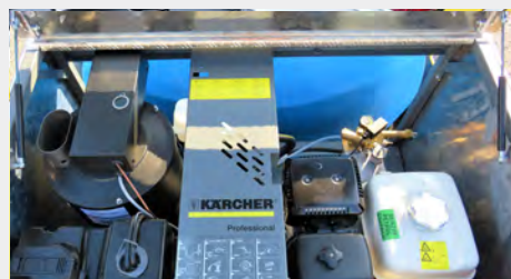
SECURE EQUIPMENT CABINET, HOUSING PUMP AND HIGH-OUTPUT BURNER WITH UPRIGHT COIL
