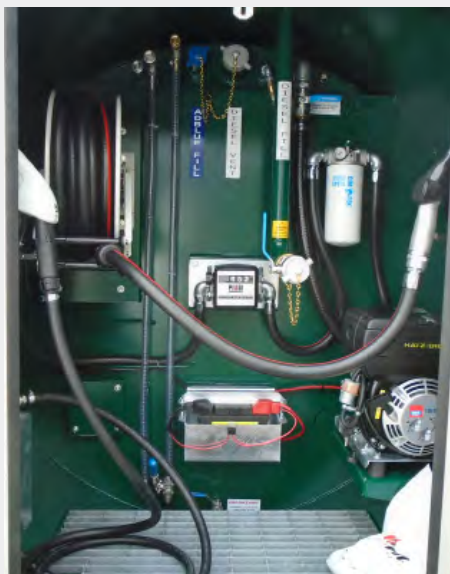
SECURE CABINET HOUSES TANK CONNECTIONS AND DUAL DISPENSING SYSTEMS FOR DIESEL & ADBLUE
