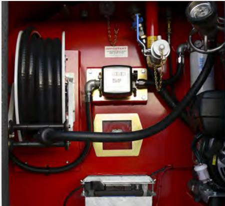
FULL-HEIGHT CABINET ON ALL MODELS ALLOWS FOR EASY ACCESS TO FUEL DISPENSING EQUIPMENT
