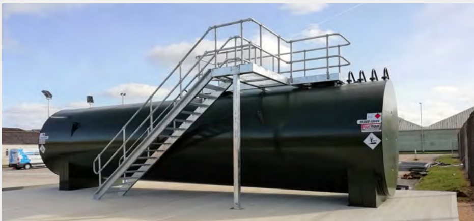
HORIZONTAL BULK DIESEL TANK WITH GALVANISED ACCESS PLATFORM
