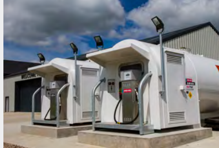
15,000 LITRE JET A-1 AND AVGAS BULK TANKS
