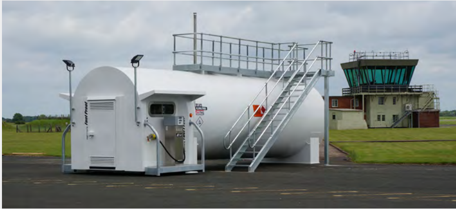
42,000L PREMIUM BULK JET A-1 TANK MANUFACTURED AND INSTALLED AT LEEDS EAST AIRPORT
